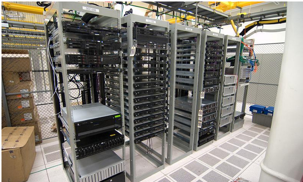
Obr. 1 – servery v racku
